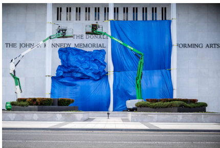
A tarp covers construction on the building's facade on Dec. 19, 2025, after Trump announced The John F.
